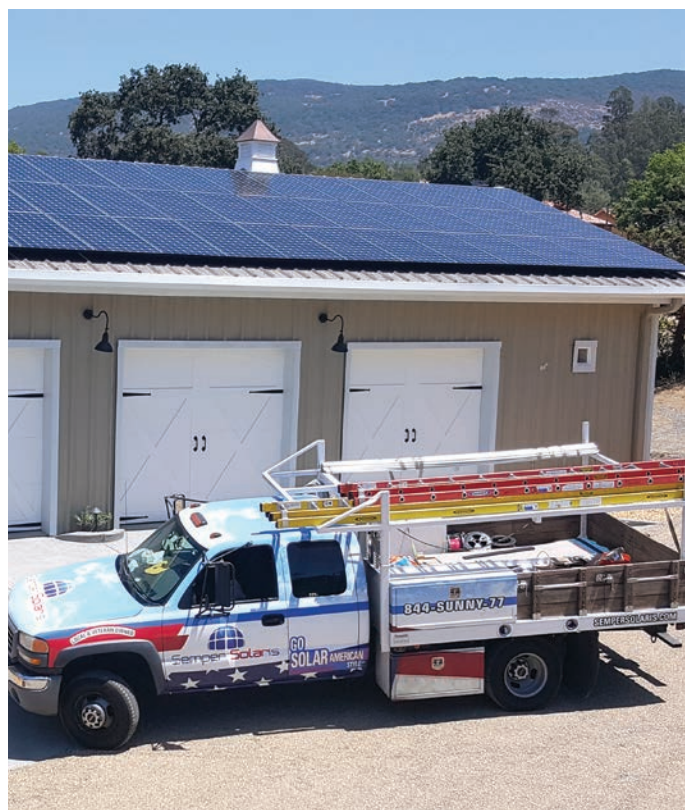
Actual SunPower installation by Semper Solaris.
